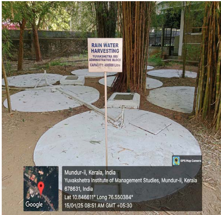
Rain water harvest at Administrative Block
